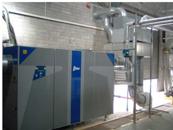
Figure 10: View on Unit and Air-Air Heat Exchanger
