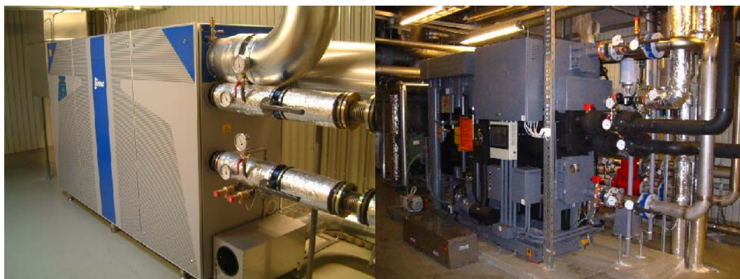
Figure 4: The Microturbine and Chiller Installation at Statoil, Stavanger
