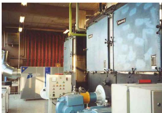
Figure 2: Two T-100 CHP Units installed in Heating Station West at Copenhagen Airport
